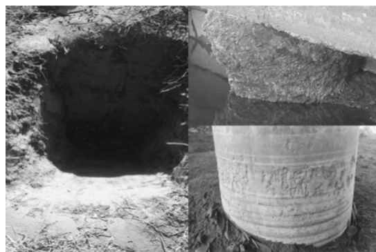
a. Soil sample taking site b. Concrete corrosion condition Fig. 1. Site collection of soil samples and situation of concrete corrosion
